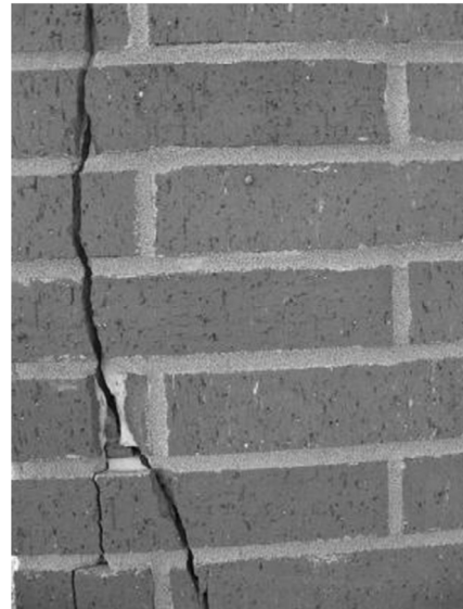
Crack due to thermal stress
